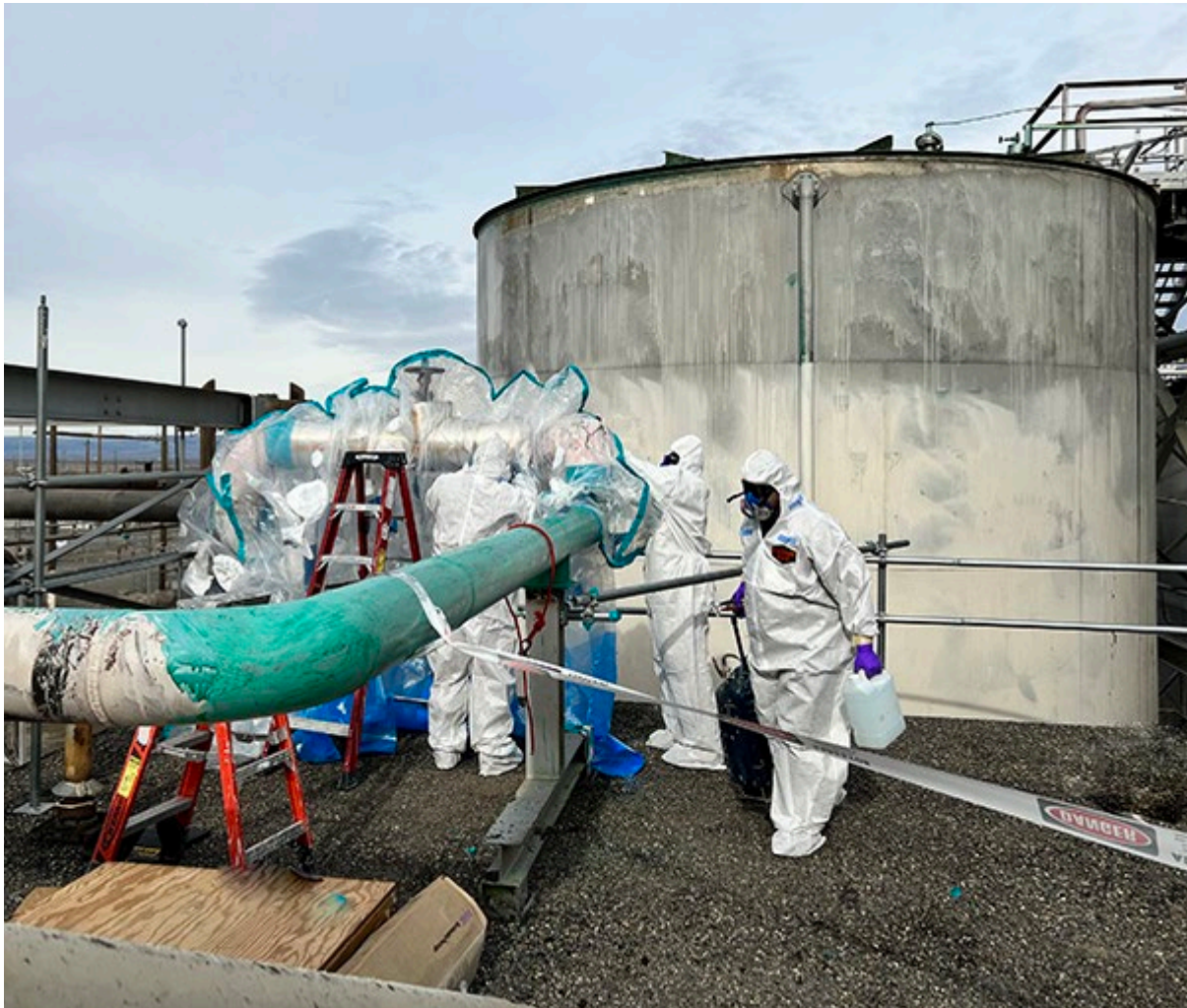
Crews remove asbestos from the 211A Pump House that supported the PUREX facility during the Hanford Site operations to allow for safe demolition of the structure.
